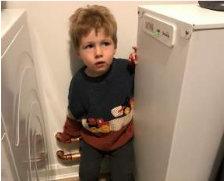
Pipes not insulated
