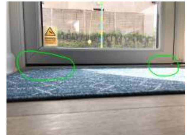
All Patio doors badly fitted or not fit for purpose
